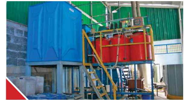
In 2025, the company successfully completed the installation of a wastewater treatment plant (WWTP), which is now operating optimally, demonstrating its commitment to sustainability and environmental compliance.
