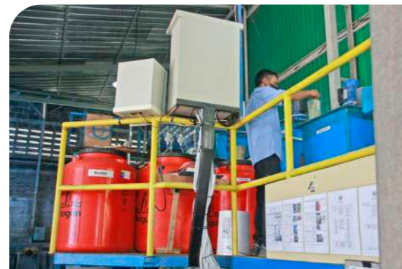
In 2024, the company successfully completed the installation of a wastewater treatment plant (WWTP), which is now operating optimally, demonstrating its commitment to sustainability and environmental compliance.
